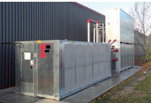
09 Installation BRW + SIREG. Circuit moule 15° + circuit huile 25° ROWENTA 27
